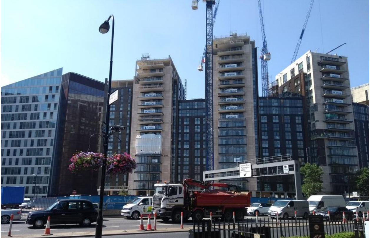
View of site from north side of the Westway (A40) – site in foreground in front of residential blocks under construction.
